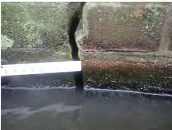
Foto 03: Detail verticale scheur
